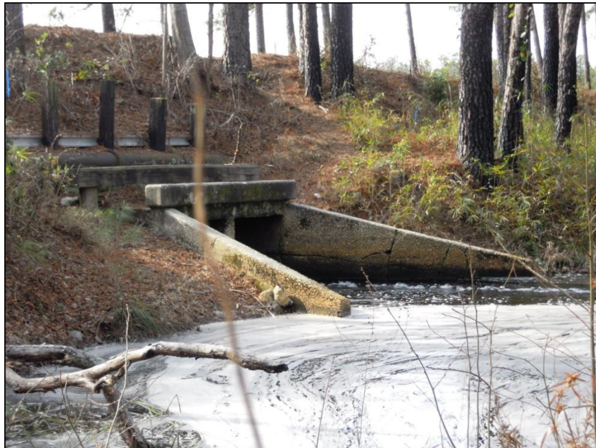
Figure 10. The spillway outlet structure consists of a two-cell, concrete box culvert. Note the partially exposed cast iron, wastewater pipe running across the embankment, just above the outlet.
