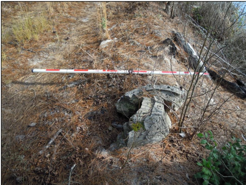
Figure 14. This manhole structure, located on the crest of the dam, has significantly deteriorated.
