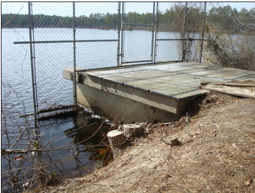
Figure 8. Modern decking and fencing have been added to the spillway intake structure. Horizontal marks left from the concrete forms used in building the drop inlet can be seen on the sides of the inlet.
