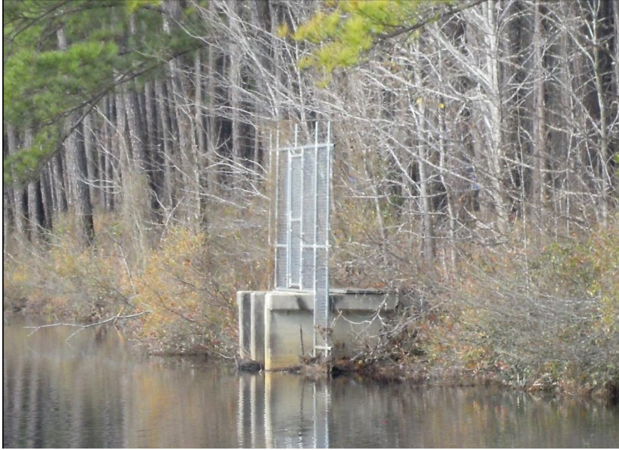
Figure 7. The spillway intake structure of the dam from the southeastern bank of the lake.
