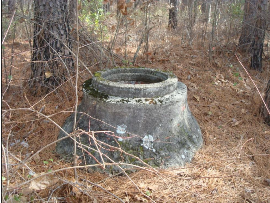
Figure 13. This is the only completely intact brick and mortar manhole structure. It is located just the southeast of the dam embankment.
