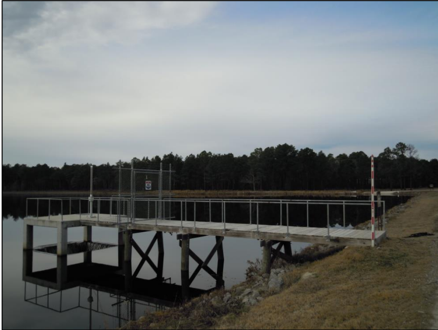
Figure 15. Work to replace the spillway inlet structure on Big Muddy Lake Dam was completed in 2009.
