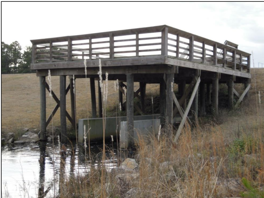
Figure 16. Work on Big Muddy Lake Dam in 2009 included replacement of the outlet structure. Note the new concrete wingwalls and observation platform.
