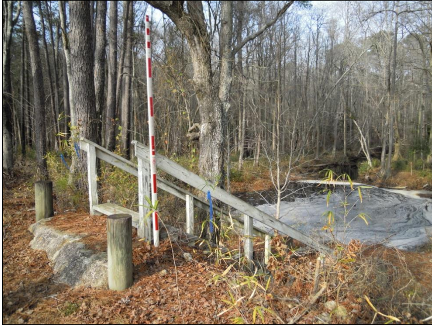
Figure 9. A set of steps leads to the spillway outlet. The concrete and stone landings at the top of and bottom of the steps are likely original; however, it appears that the wood steps and railings have been replaced.
